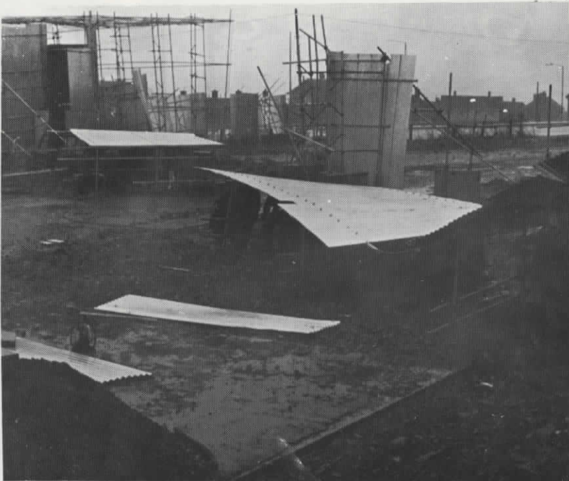
Storm damage at the new Whiterock Base.
